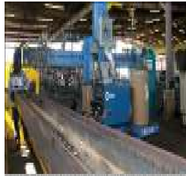
The fixed automation system, which uses mechanical hardwired logic to perform a series of tasks, is typically used in the production of high-volume, low-variety products.
